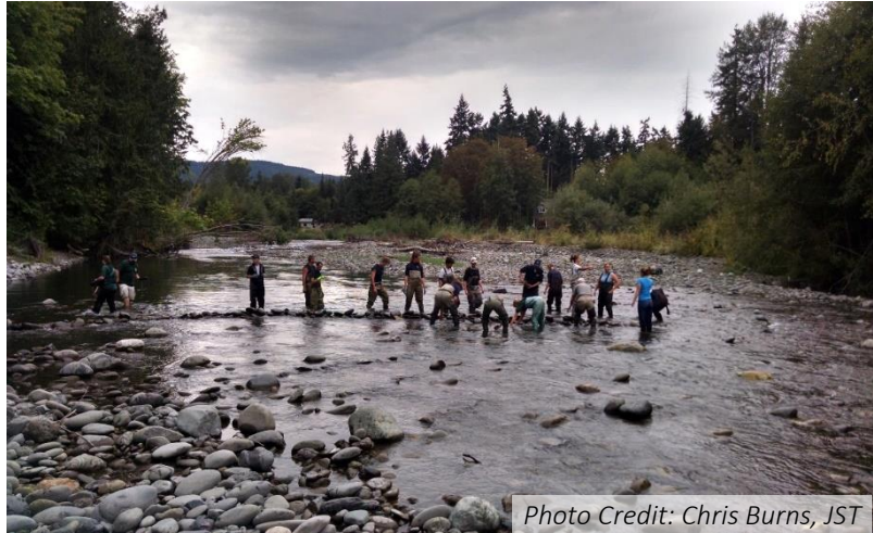
Crews installing rock dams in the Dungeness River to help fish move upstream during the 2015 Drought.
