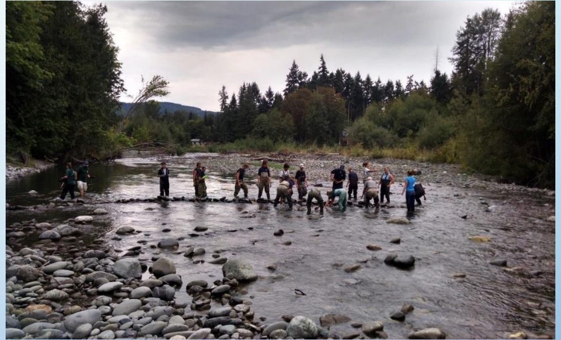
Crews installing rock dams in the Dungeness River to help fish move upstream (2015 Drought).
