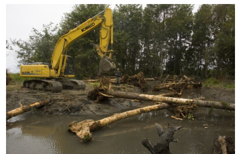
Logjam being constructed in a side-channel of Dungeness River. Photo by Tiffany Royal.
